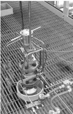
FIGURE 6: INSTALLED TAIL GAS PROBE AND FIBER OPTICS GOING BACK TO THE ANALYZER (PATENT- PENDING)
